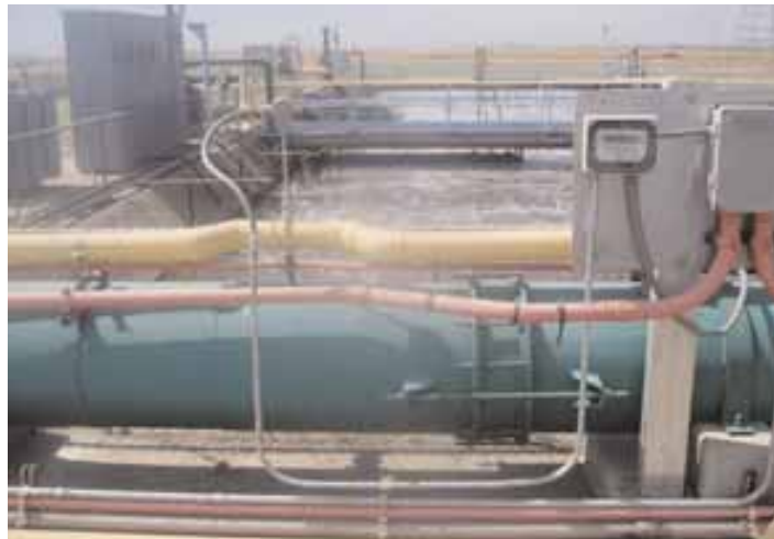
Thermal meter monitors wastewater treatment plant blower airflow rate.
