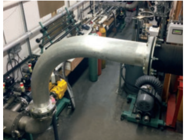
Main Intake to High Velocity Facility
